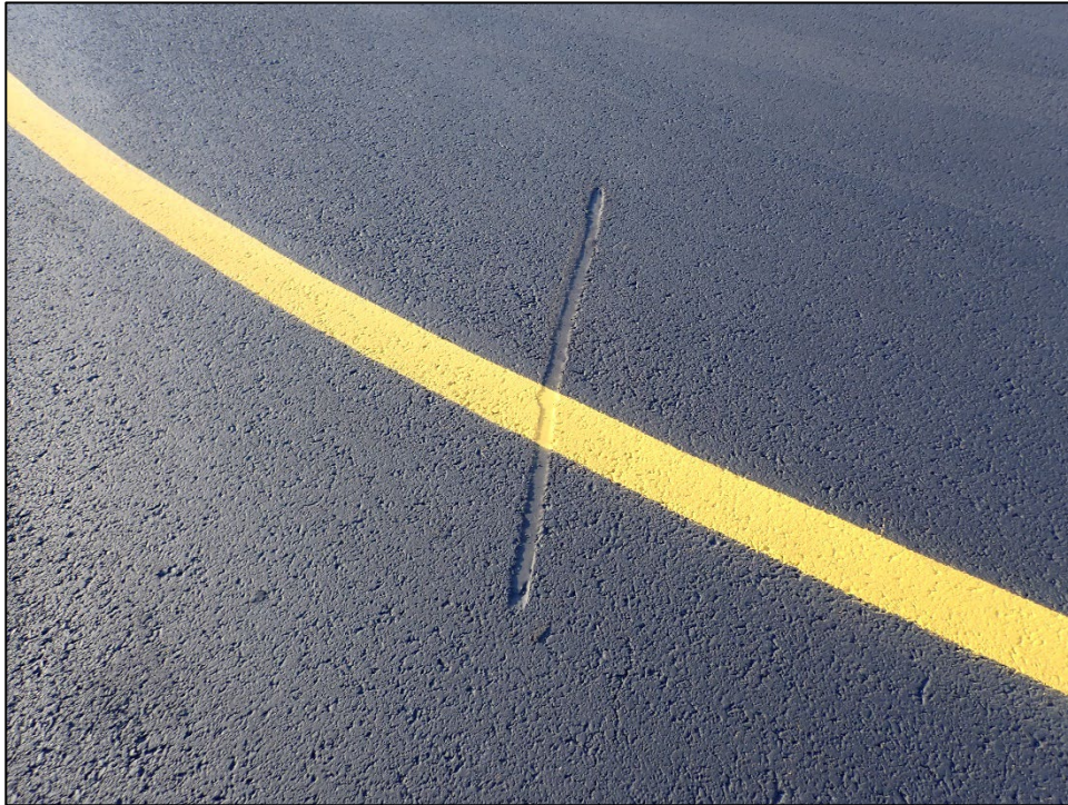
TW-04-01: L&T Cracking
