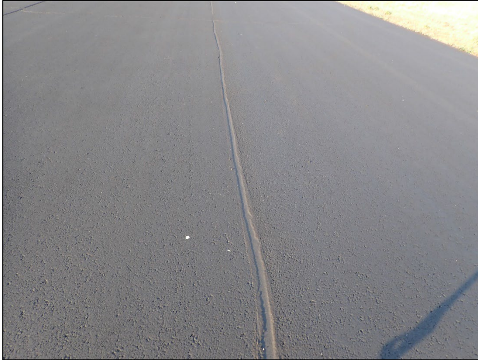
RW04-02-44: L&T Cracking
